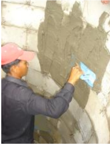
Figure 13 - Applying the first layer of render to the inside of the tank
